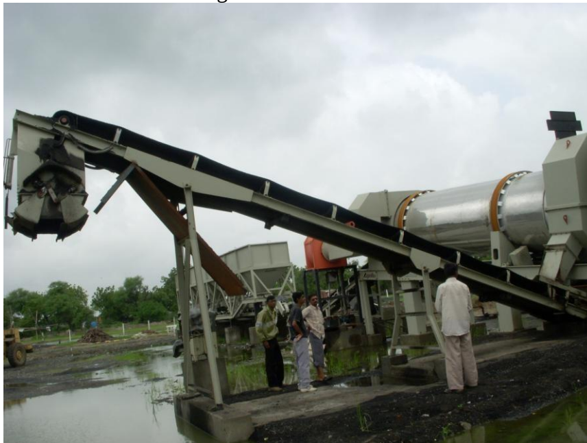
Fig. Load Out Conveyor
