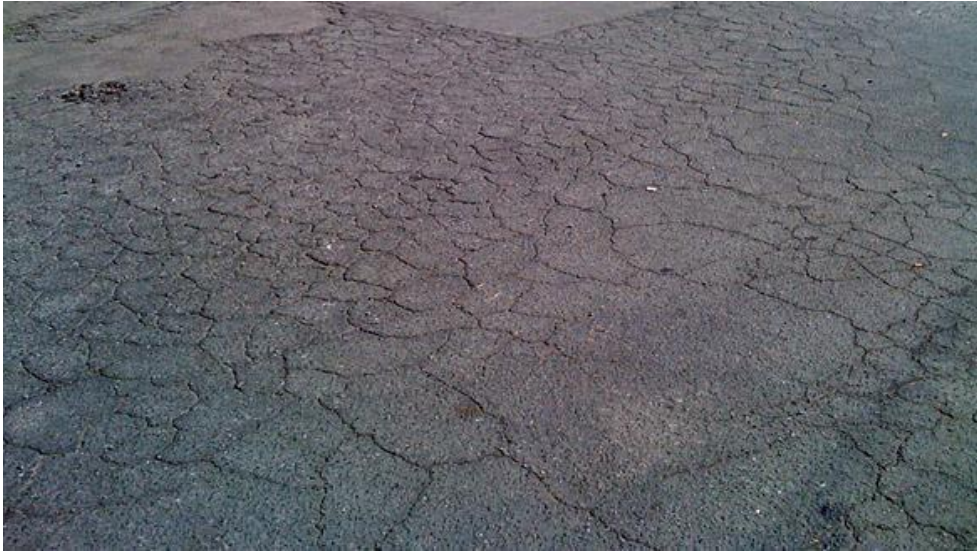
Fig. Alligator Cracking
