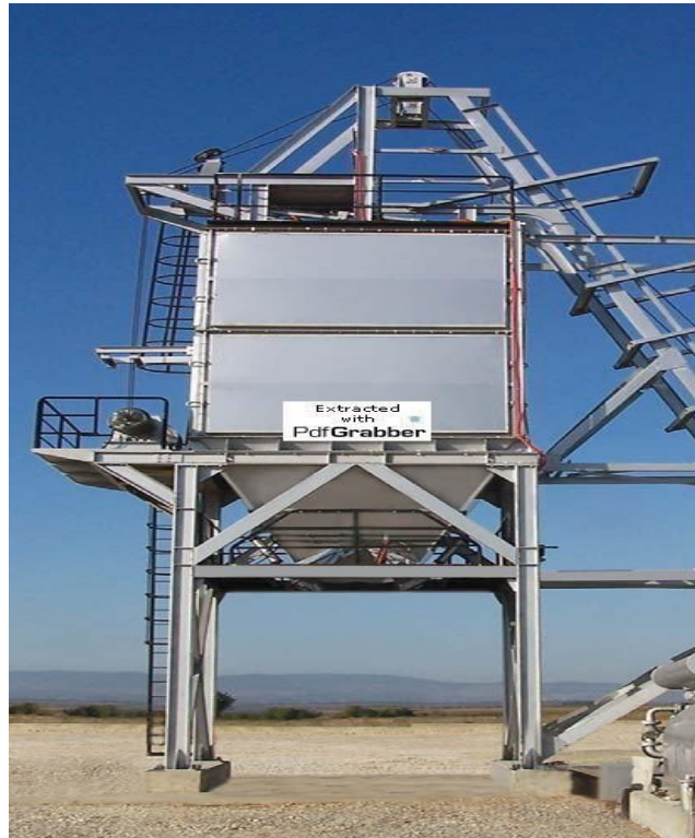
Fig.Hot mix storage silo
