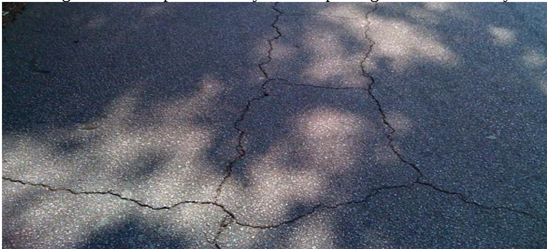
Fig. Block Cracking
