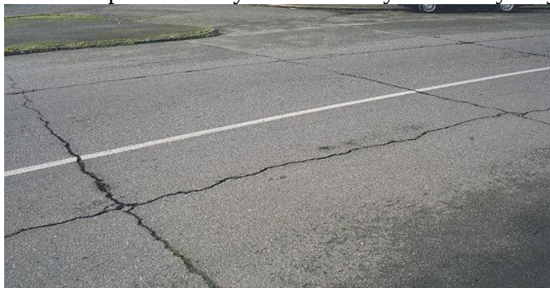
Fig. Joint Reflection Cracks
