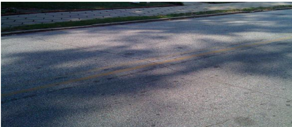
Fig. Transverse Cracking
