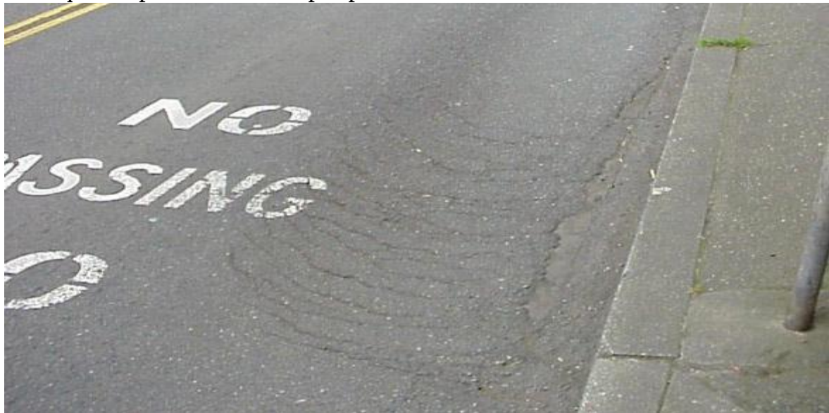
Fig. Slippage Cracks
