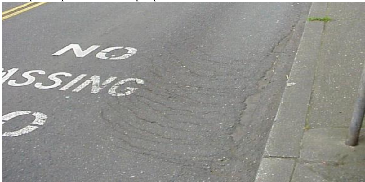
Fig. Slippage Cracks
