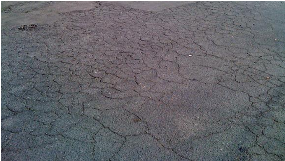
Fig. Alligator Cracking
