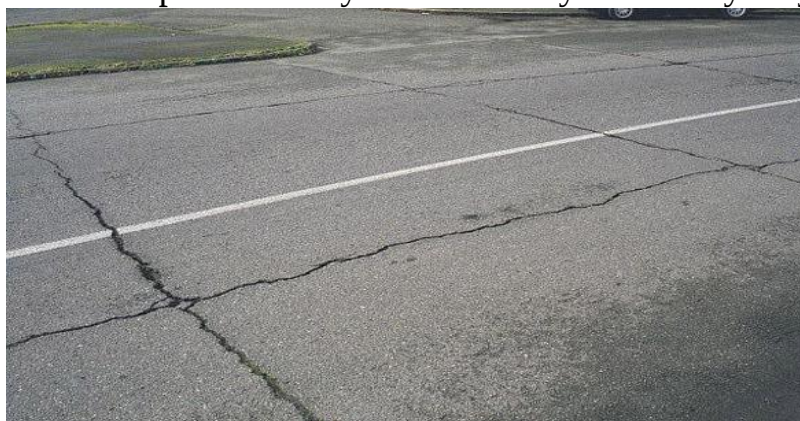
Fig. Joint Reflection Cracks
