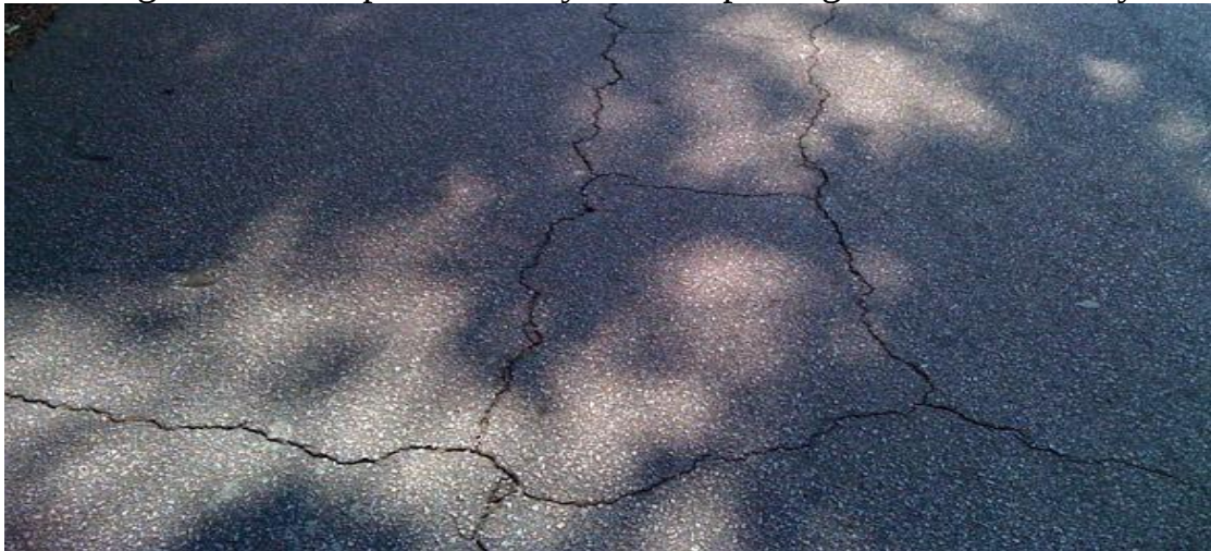
Fig. Block Cracking
